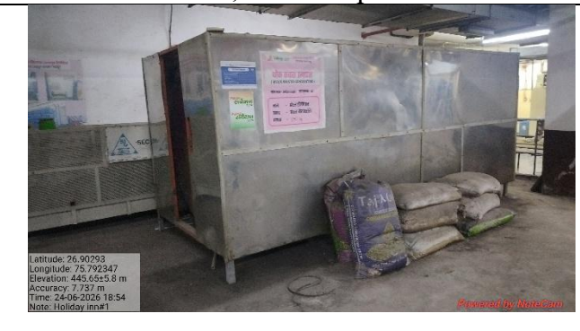
Organic waste Compost machine at Holiday Inn
